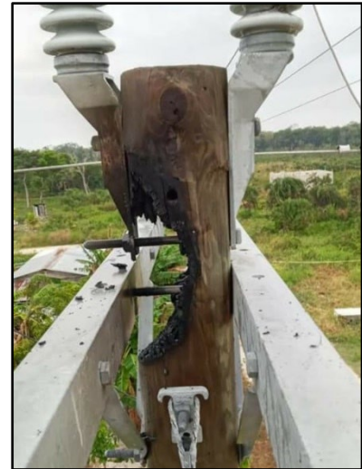
Burnt pole top due to higher than expected dust build-up.
